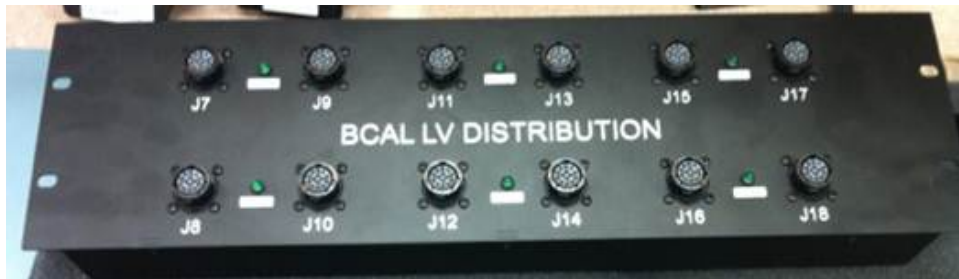
Figure 3.77: LV distribution chassis
